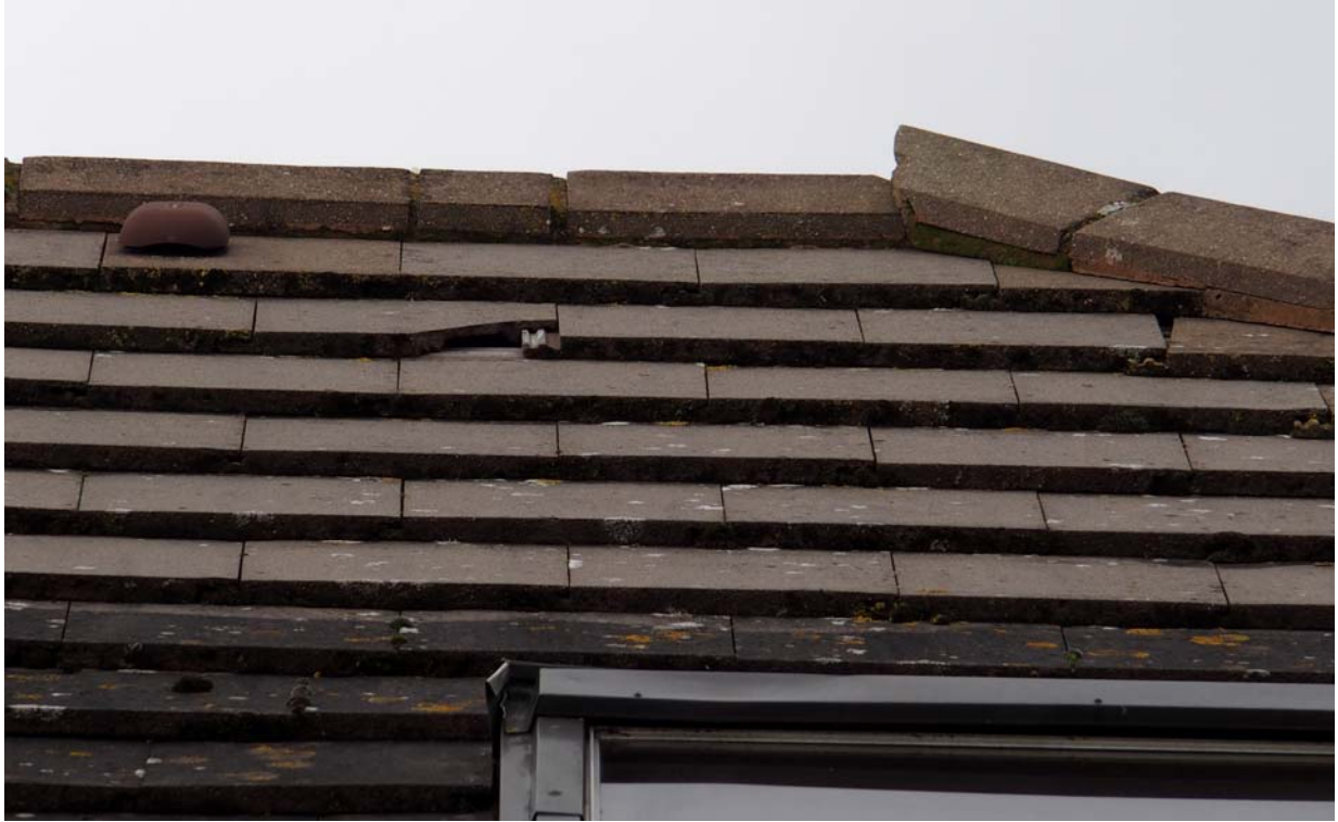
Photograph No. 07 - 2 no. potential access points. Upon further internal inspection these access points were discounted.
